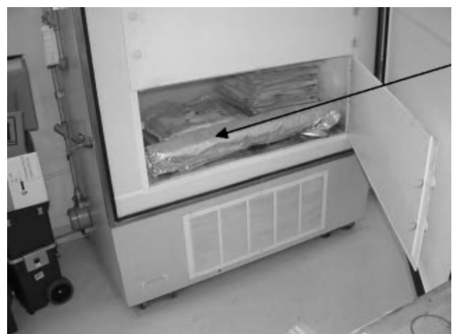
Figure 10 – Rotodome bearings in cold chamber
